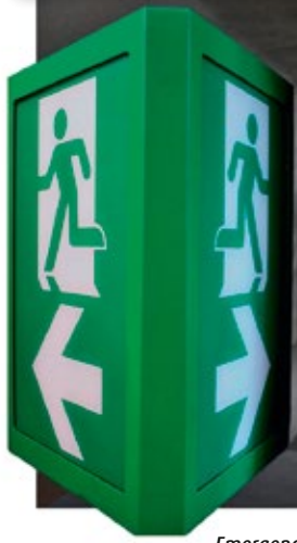
Emergency and safety lights in the Ceneri Base Tunnel
